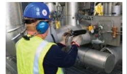
LEAK LOSS AUDITS
